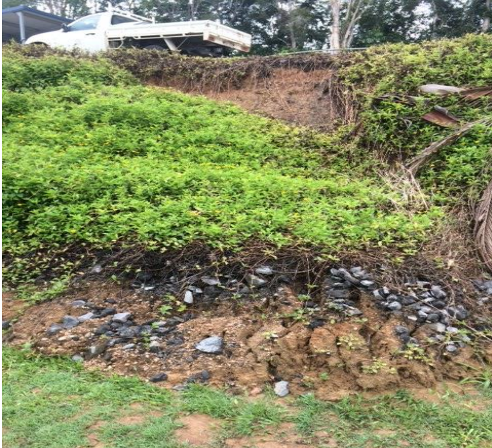
Kuranda WWTP embankment slip
