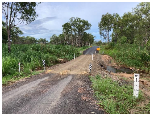
Temporarily repaired causeway – Carman Road
