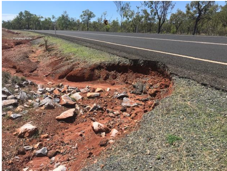
BDR shoulder scour – Ch 564 to Ch 579
