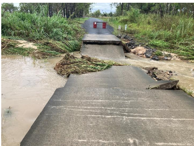
Failed causeway – Carman Road
