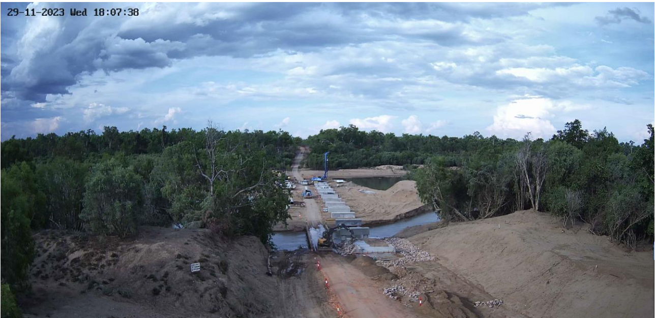
Gamboola Crossing over Mitchell River, Strathleven Road – construction of bridge piers and headstocks in progress
