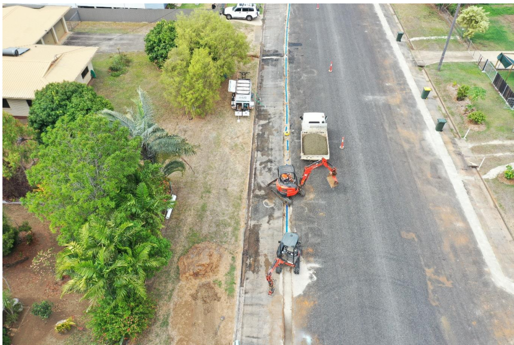
Mason Street installation of the new 150mm diameter PVC Supermain water main
