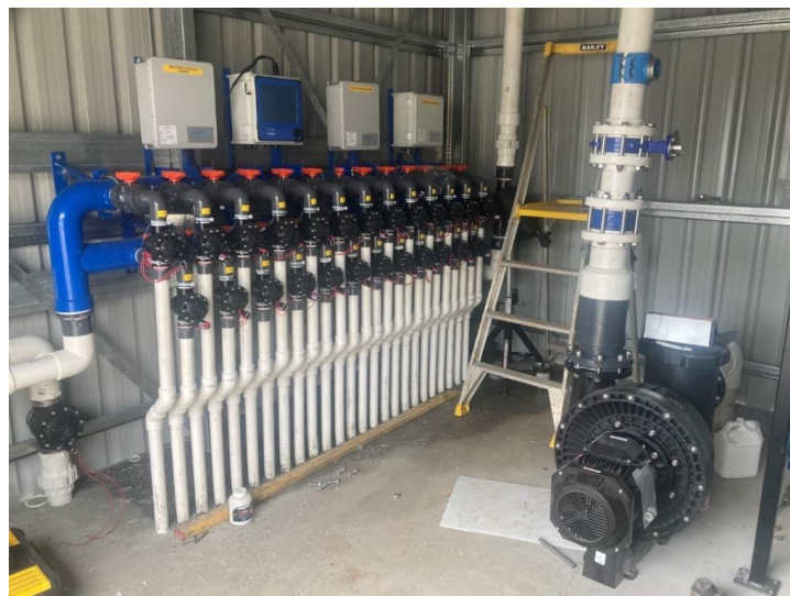
Splash Park Filtration Shed
