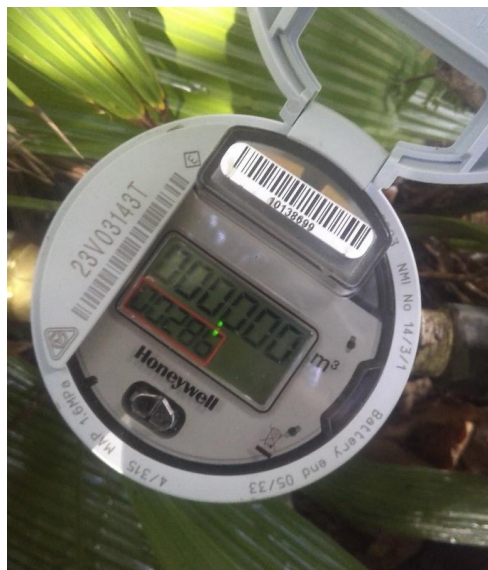
A new fully integrated smart meter that was recently installed in Kuranda.
