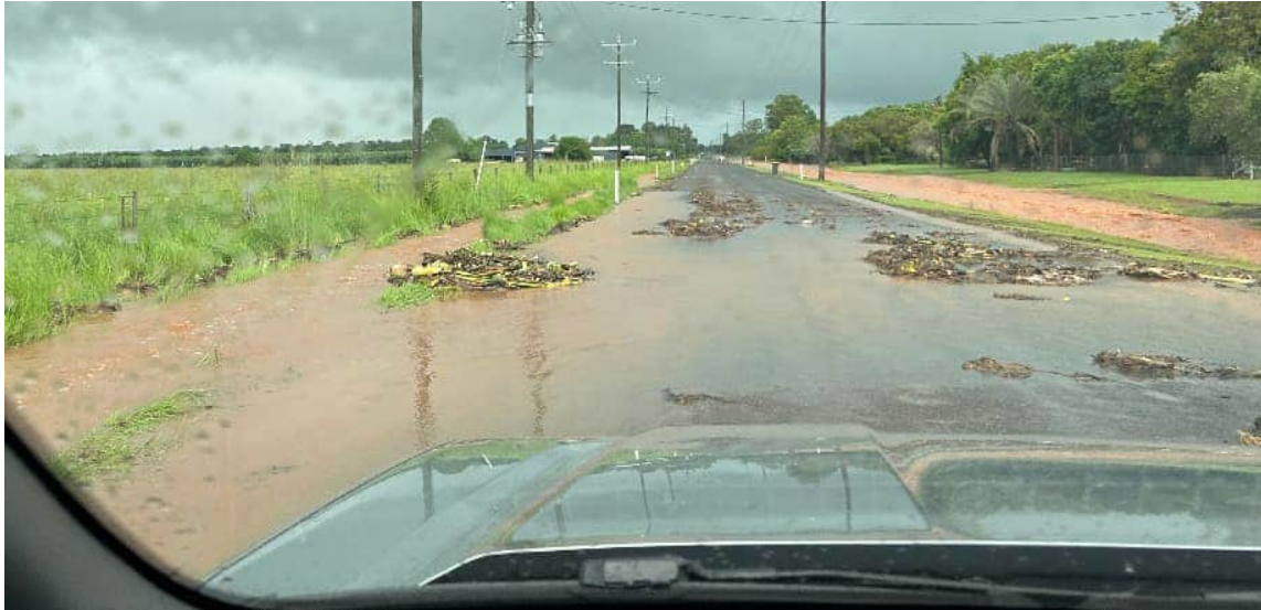
Figure 5: Example of Runoff Overtopping Ray Road Due to Exceeded Drain Capacity (Heading North on Ray Road, Just north from George Fabris Road, 22 December 2024)
