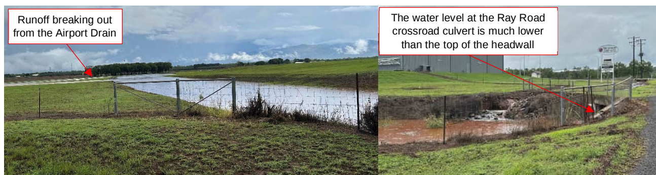
Figure 14: Example of Runoff Exceeding the Capacity of the Airport Drain (Looking East from Ray Road)
