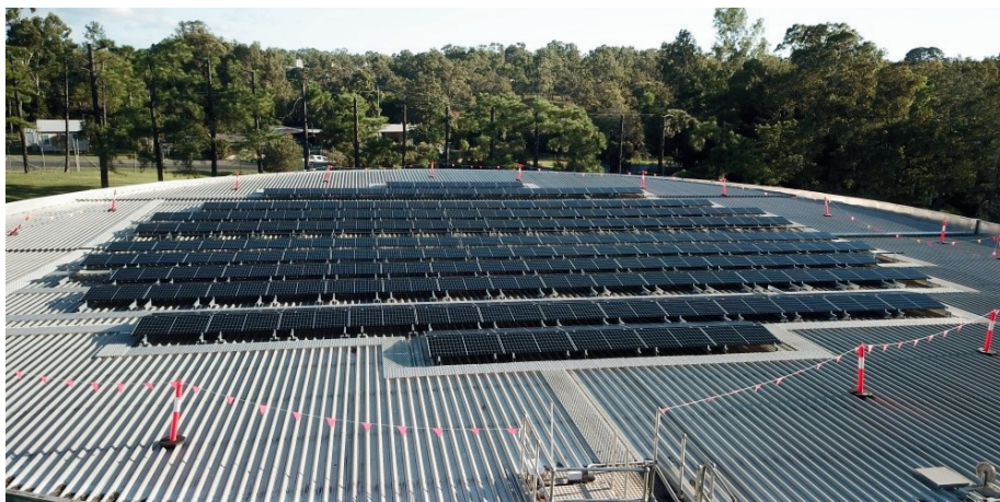
Solar installation Mareeba water treatment plant
